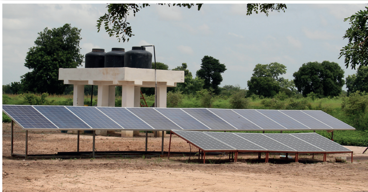
Solar powered borehole
